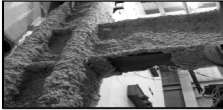
Figure 1. The collapse of fire insulation cover in place of plastic hinge [12]
