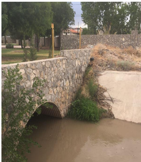
Image 10 Ditch taken advantage of in a fractionation to the south east of the city. Own image 07/2020
