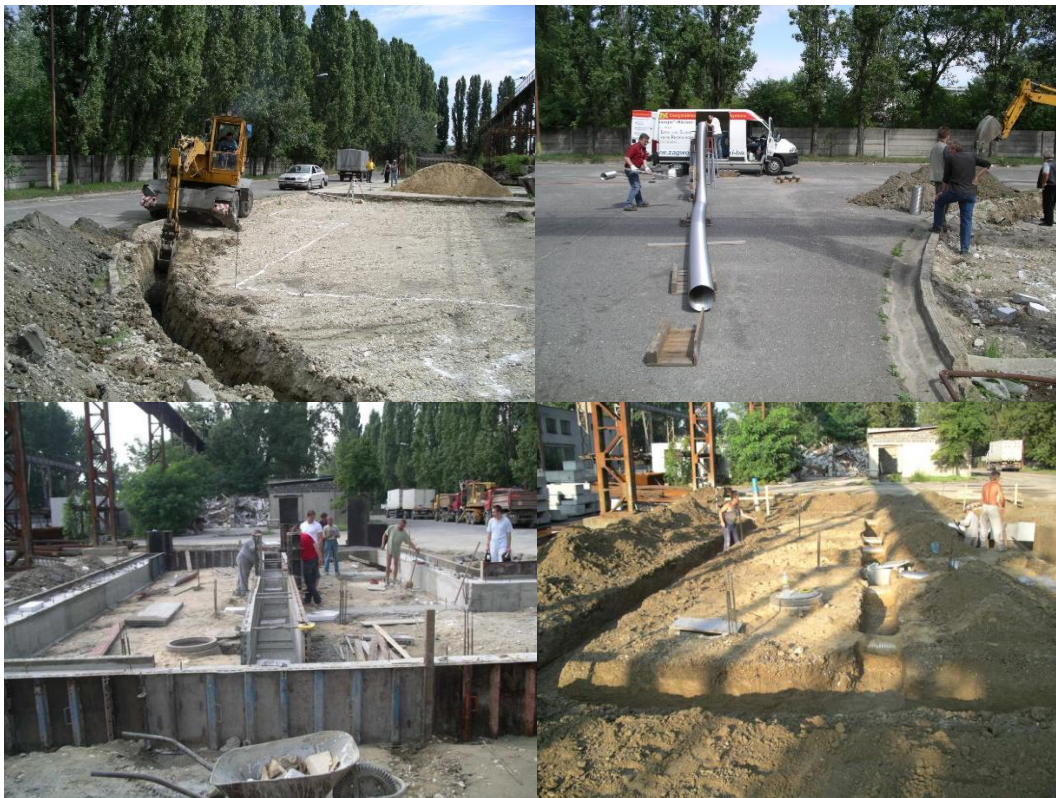
Figure 9: Photos of excavations and installation of a recuperative ground heat exchanger used for recuperation ventilation of the type panel house IDA I. (photo archive: Kalús, D.) [7, 8, 9]
