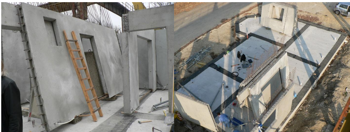
Figure 2: Manufactured reinforced concrete panels of the type panel house IDA I. (photo archive: Kalús, D.) [7, 8, 9]
