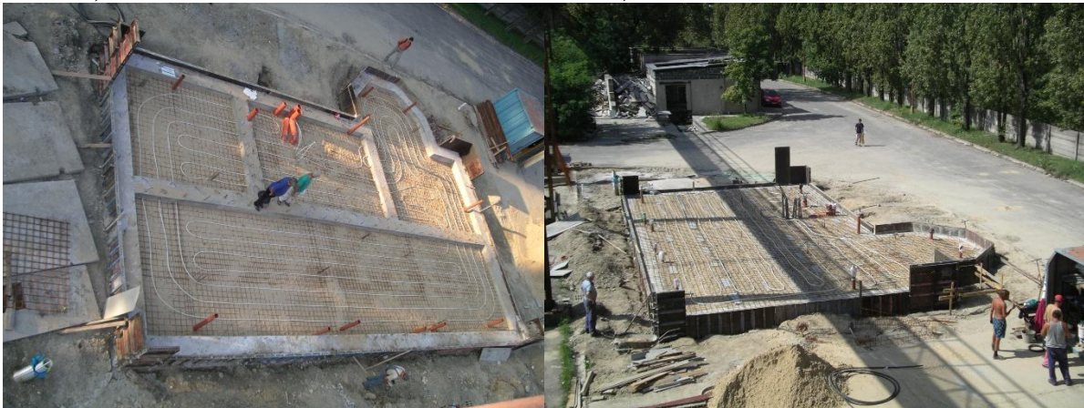
Figure 7: Circuit in GHS above the foundation slab and directly in the foundation slab (photo archive: Kalús, D.) [7, 8, 9]
