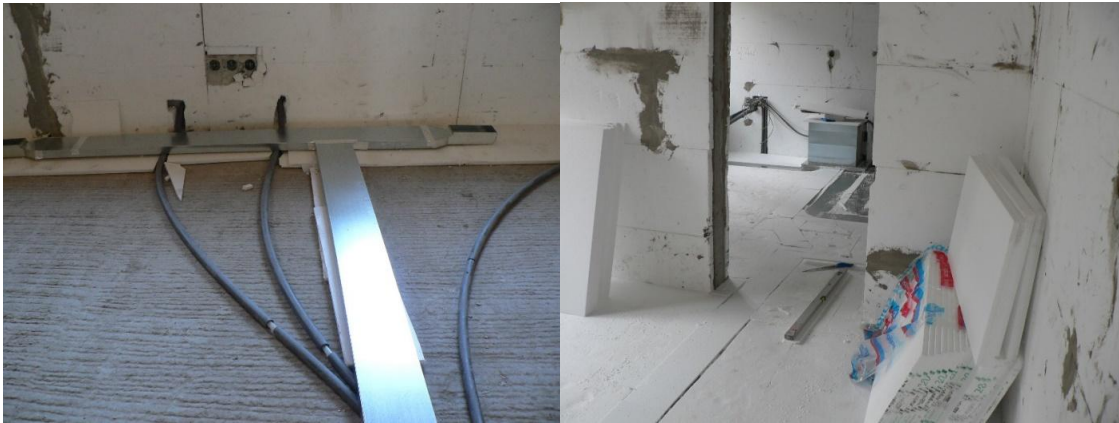
Figure 12: Installation and insulation of ventilation ducts in the interiors of the type panel house IDA I. (photo archive: Kalús, D.) [7, 8, 9]
