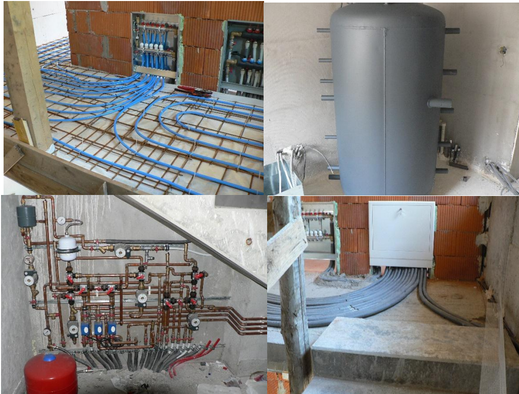
Figure 8: Photos from implementation of underfloor heating, a view of the storage tank of heating water, the engine room of energy systems and the cabinet of the distributor and the collector with the connection of ATP circuits in the circuit panels (photo archive: Kalús, D.) [7, 8, 9]
