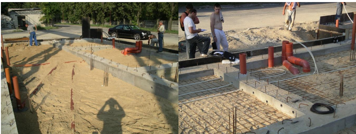
Figure 11: Distribution of ventilation ducts of the recuperation ventilation system under the foundation slab of the type panel house IDA I. (photo archive: Kalús, D.) [7, 8, 9]
