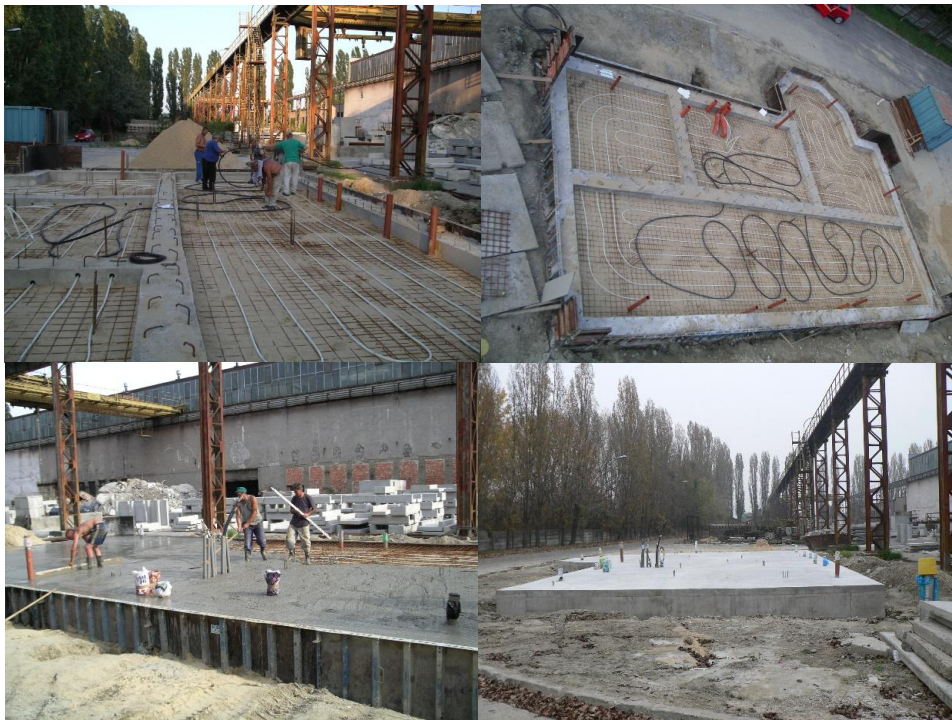
Figure 13: Installation of pipes for preheating hot water in the ground heat storage built-in under and in the foundation slab of the type panel house IDA I. (photo archive: Kalús, D.) [7, 8, 9]
