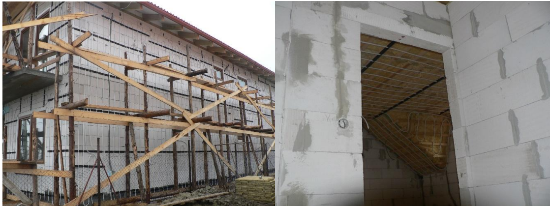
Figure 5: View of the ATO formed by a plastic pipe between aerated concrete masonry (375 mm) and EPS (100 mm) and in the construction of the roof in circuits: 20 x 100 m in the experimental house EB2020 (Photo archive: Kalús) [10, 13]
