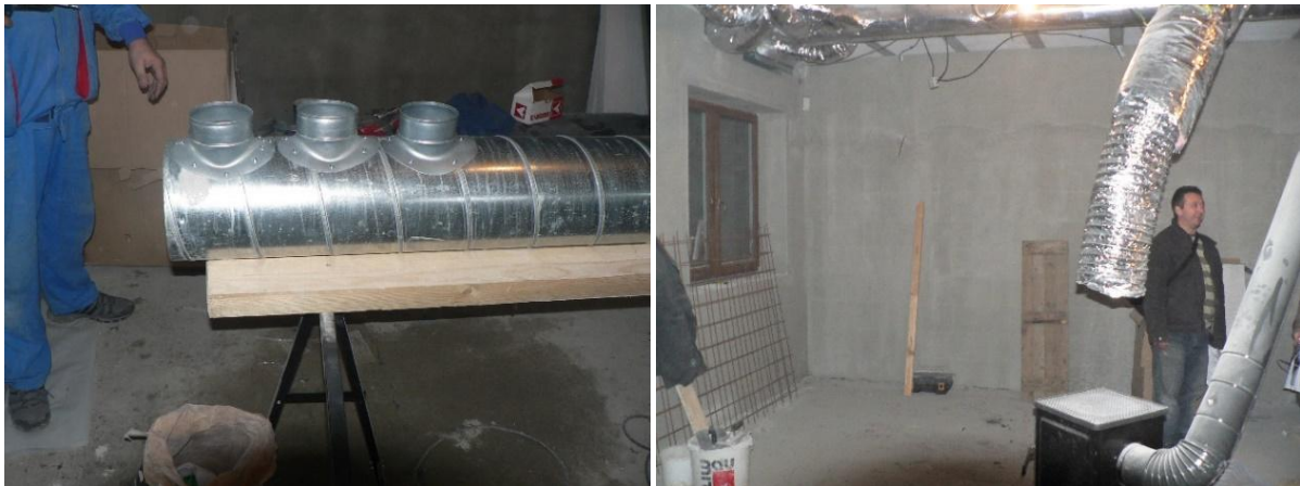
Figure 8: View of the implementation of recuperative ventilation in the experimental house EB2020 (Photo archive: Kalús) [10, 13]
