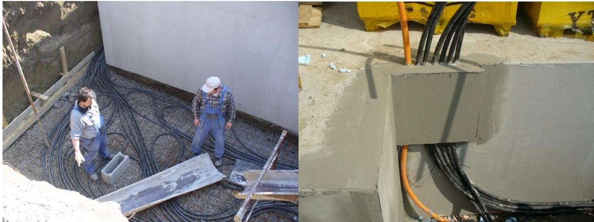
Figure 6: View of cooling circuits, which are located in the non-freezing depth, in the ground around the foundation strips of the building in the experimental house EB2020 (Photo archive: Kalús) [10, 13]
