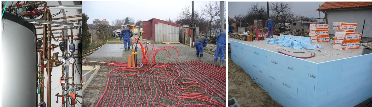
Figure 4: View of the storage tank ( V = 575 l for CH and 180 l for DHW), implementation and insulation of the ground heat storage with integrated pipes in the foundation slab (Photo archive: Kalús) [10, 13]
