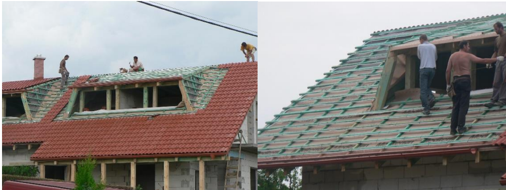
Figure 6: A view at implementation of the energy roof at the experimental house in Tomášov (Photo archive: Kalús) [10, 13]
