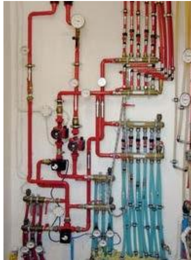
Figure 2: View of the technical room with the installed energy system with ATP, energy roof, and ground heat storage [2, 20, 41]
