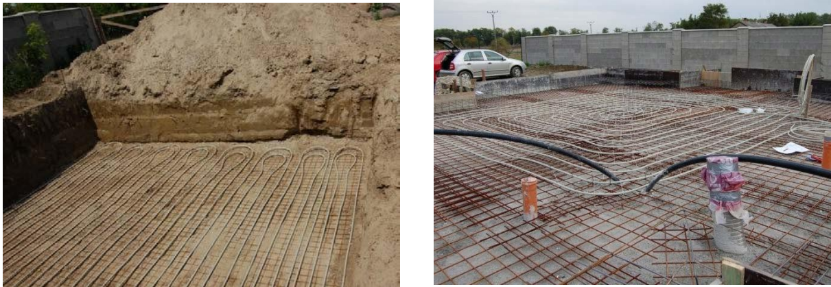
Figure 1: Construction of horizontal ground heat storage, which consists of exchangers formed by plastic pipes [60]
