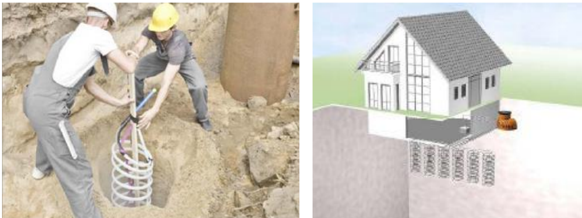
Figure 2: Construction of vertical boreholes that can be used to store and remove heat from the ground. Pictured on the right used for a heat pump [58]
