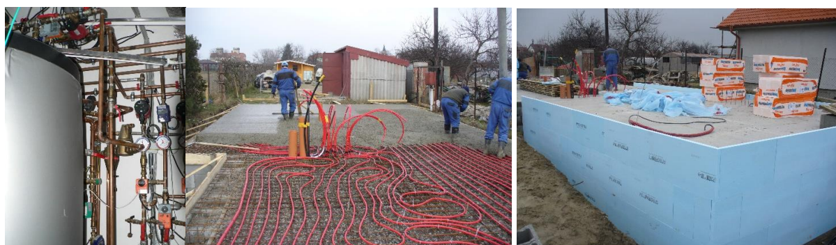
Figure 9: View of the storage tank ( V = 575 l for CH and 180 l for DHW), implementation and insulation of the ground heat storage with integrated pipes in the foundation slab (Photo archive: Kalús) [10, 13]
