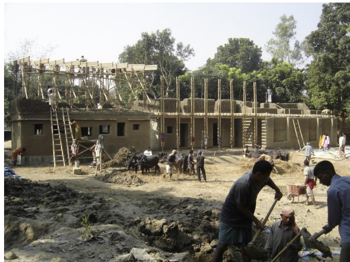
Image 11. Mud as the primary material for METI School- Bangladesh Mud as the primary material that involves community participation, easy maintainance and construction
