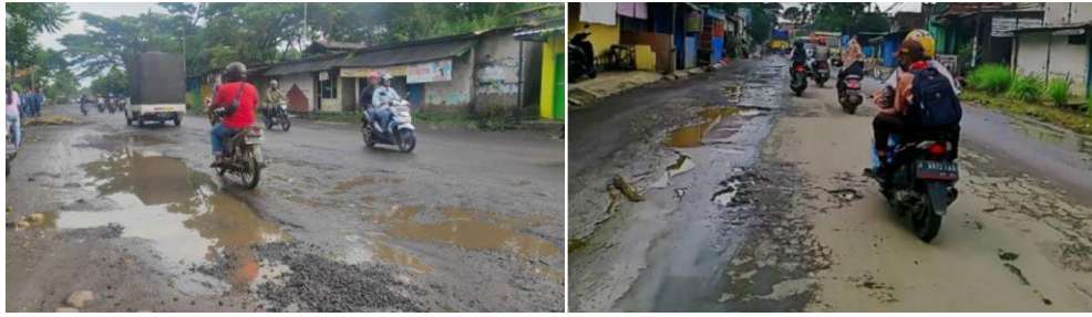
Figure 1.1 Picture of road condition of Kreet - Gondanglegi Source : Data survey(2021)
