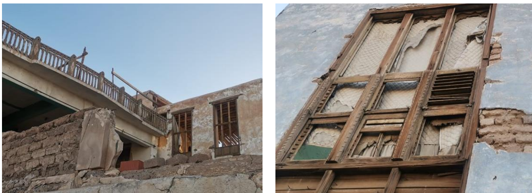
Figure 4: Peeling of Walls & Ceiling
