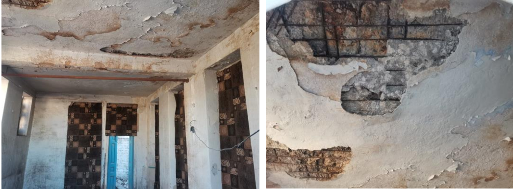
Figure 3: Roof Leakage & Mold Stains
