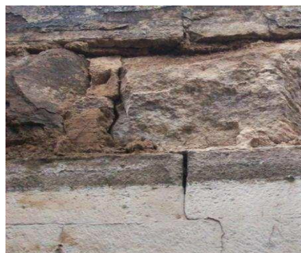
Figure 16 Vertical Cracks and Gaps.
