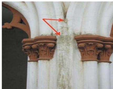
Figure 15 mold stains as the arrows showed.
