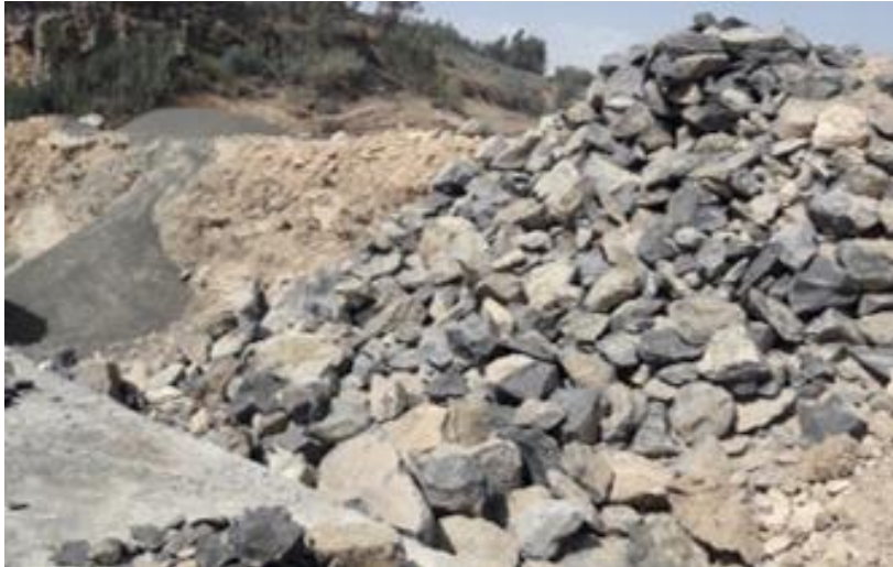
Figure 6: Poor Storage of Stone on site
