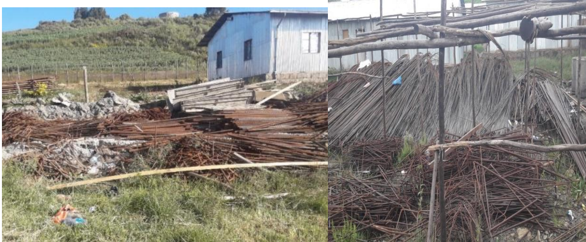
Figure 4: Wastage of Steel Reinforcement due to improper cutting of bars and design change
