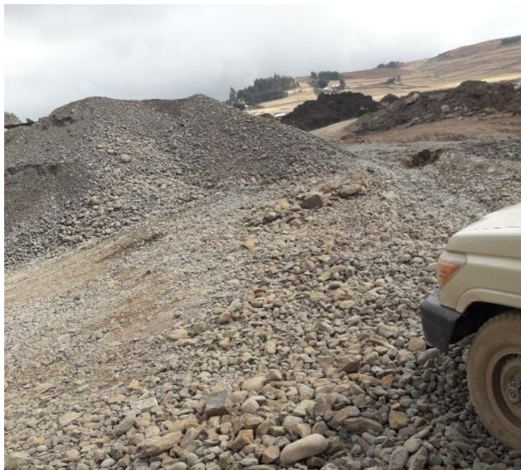
Figure 7: Poor handling of coarse aggregate onsite
