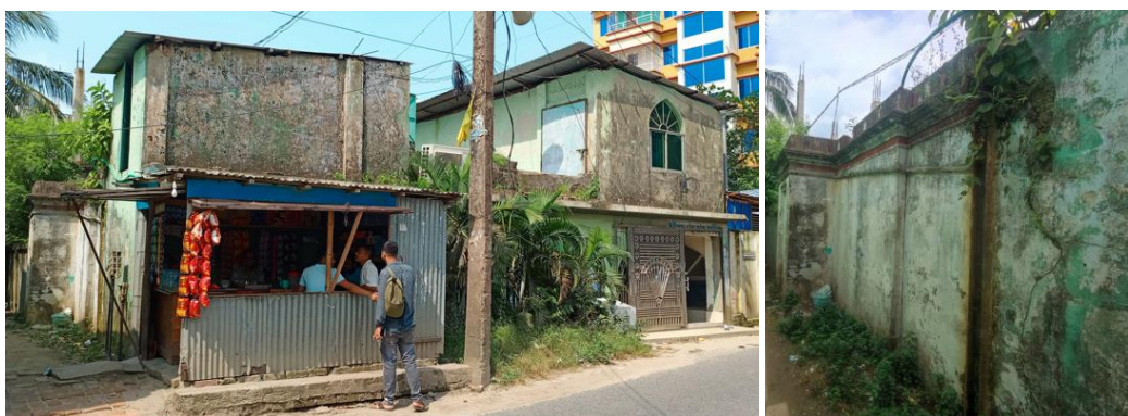
Fig.18 Present Condition of Yusufganj Mosque, It's Effects, Building Materials. Photos by, Author.
