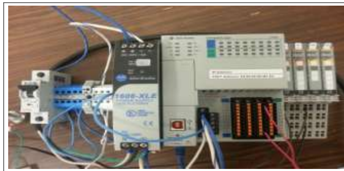
Fig 5. The PLC hardware 1769 Compact Logix controller
