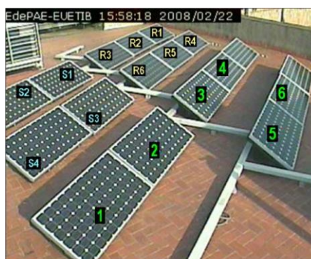
Fig. 8. Modules layout of the PV system. [R1...R6] Mention system. [S1...S4] Static section. [1...6] Reconfigurable section.
