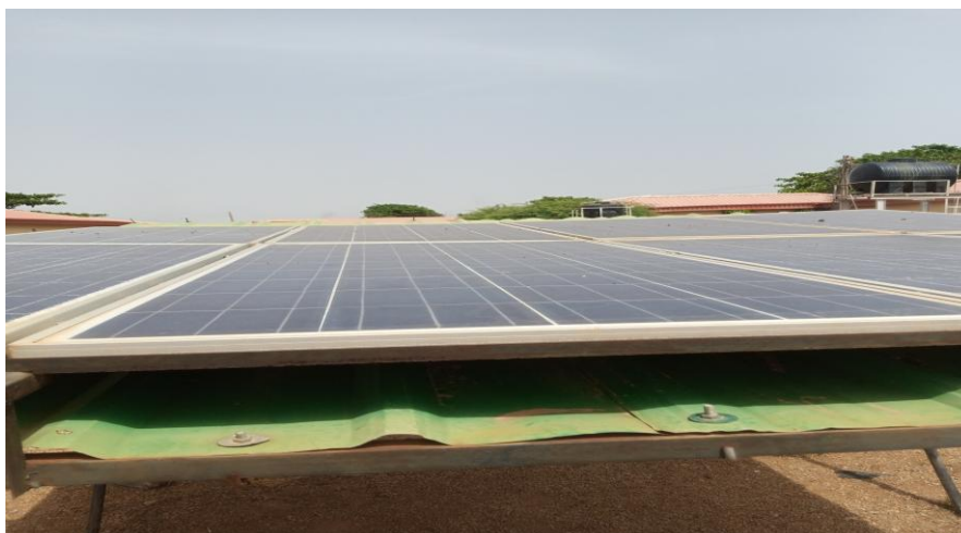
Figure 1: Solar photovoltaic panels array.
