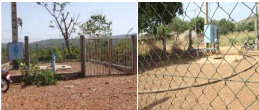
Photo assembling 3: SONEB water provision device protected with a grid fence
