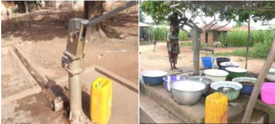
Photo assembling2: Drill equipped with motor with human force use for water extraction set up inside the Natitingou Secondary School No 1, in the Winkè area
