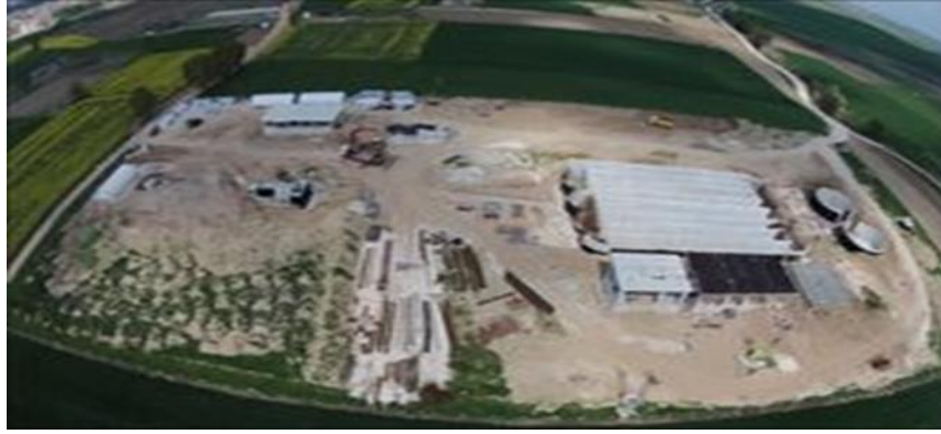
Figure 6. Babaeski Municipality waste water treatment plant [6]
