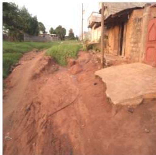
Photo 1b: Gully nearby concessions Avakpa-Kpodji neighborhood in Porto-Novo
