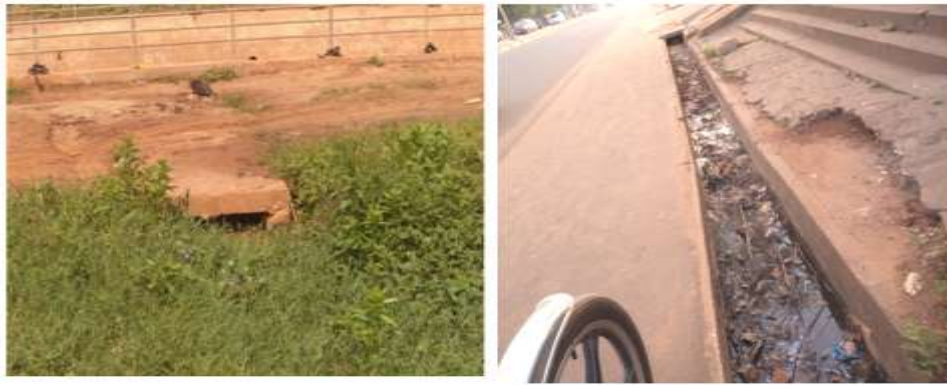
Photo 3a: Gully clogged at Kandévié
