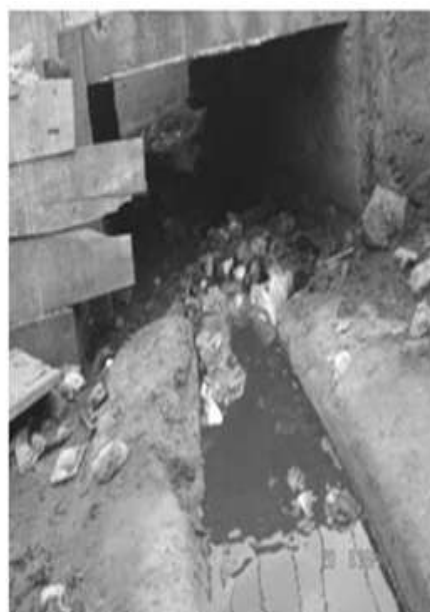
Plate2. The main drainage filled to the brim with waste fluid and solid wastes from cleaning processes.
